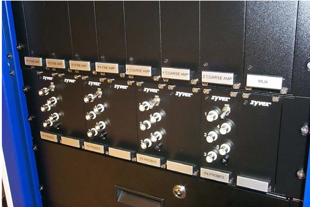
Figure 4.4. Zyvox Patch Panel Rack
